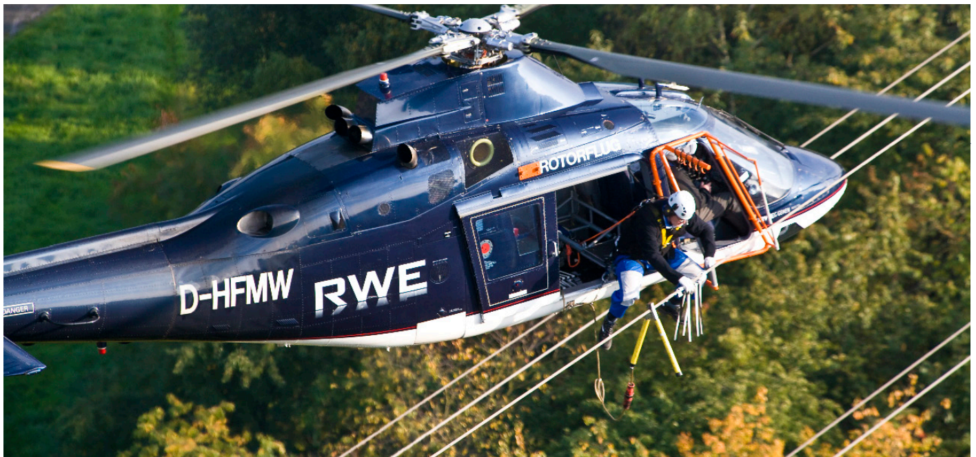
Installation of bird flight diverters by helicopter on a high voltage power line in Germany © RWE Rhein-Ruhr Netzservice
