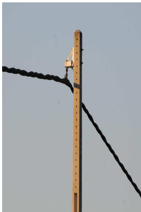
Figure 9: Completely insulated medium tension cable in Spain hanging from concrete pole without need of insulators (source: Haas, 2011).
