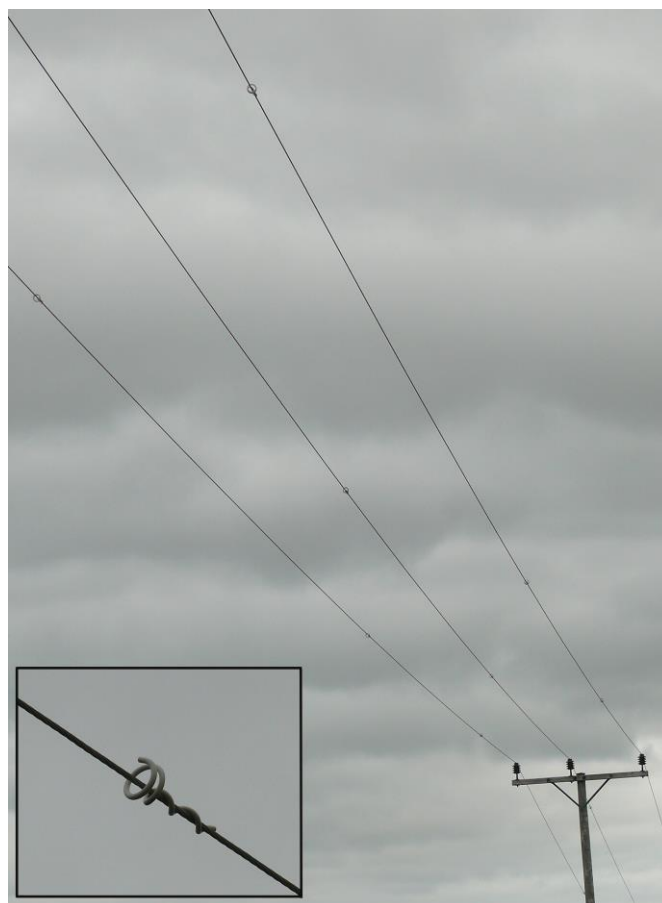
Figure 19: Medium voltage distribution line with small spirals (so-called 'pig tails') placed at regular intervals in the conductors as bird flight diverters (Photo: Bureau Waardenburg).
