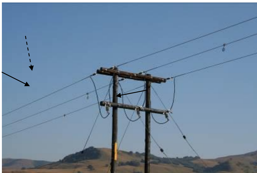
Figure 8: A safe strain pole structure, with insulated jumper wires (black arrows) and sufficiently long insulators (broken arrow) (Photo: EWT-WEP).
